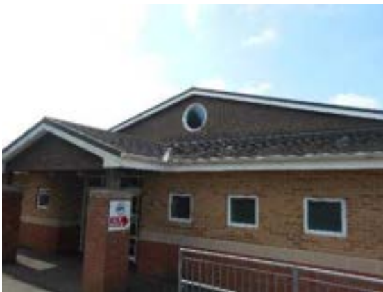
Photograph 5. Building B4 – shallow pitched roof, with tiled porch extension on the north aspect
