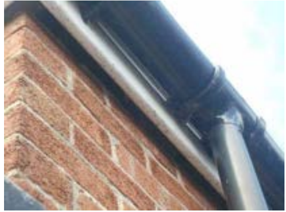
Photograph 2. Building B1 – small gaps between fascia boards and exterior wall.
